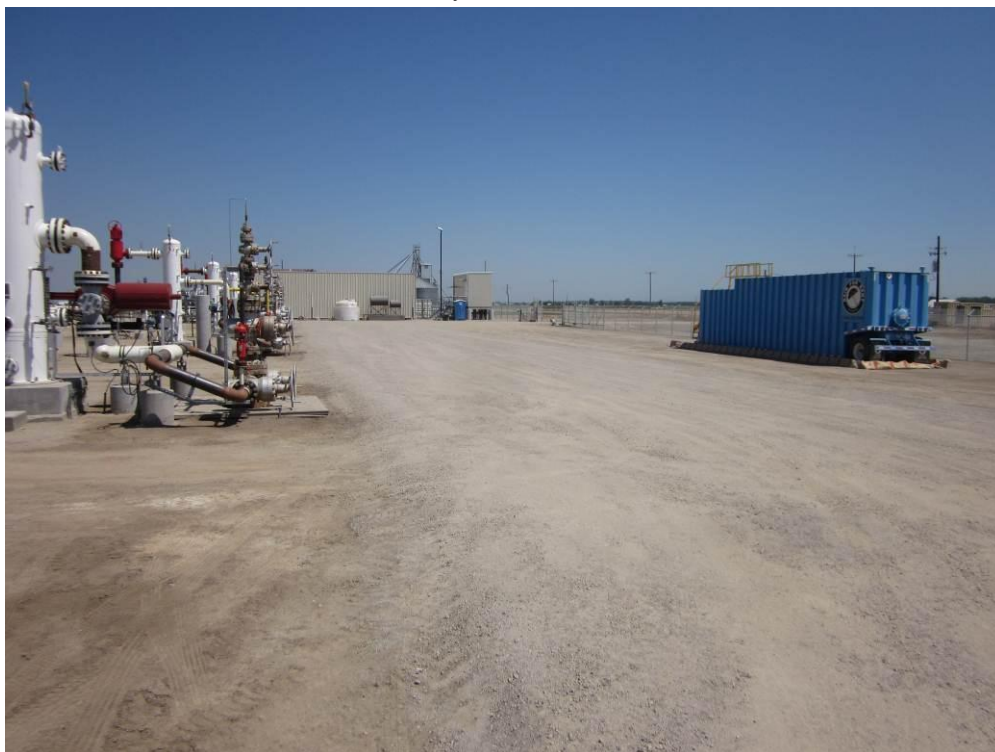
Photo 2: Materials and supplies have been removed from the Remote Well Pad site. Water tanks and temporary fluid storage systems still require removal. The final base has also been installed.
