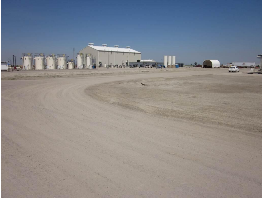
Photo 5: The compressor building has been completed and the seven fluid storage tanks (left) have been installed at the Compressor Station site. Electrical work at the fluid storage tanks was underway.
