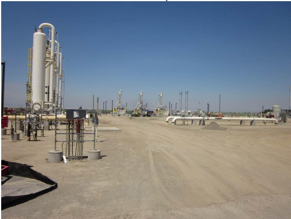
Photo 6: The dehydration towers (left) and reboilers (center) have been installed at the Compressor Station site.
