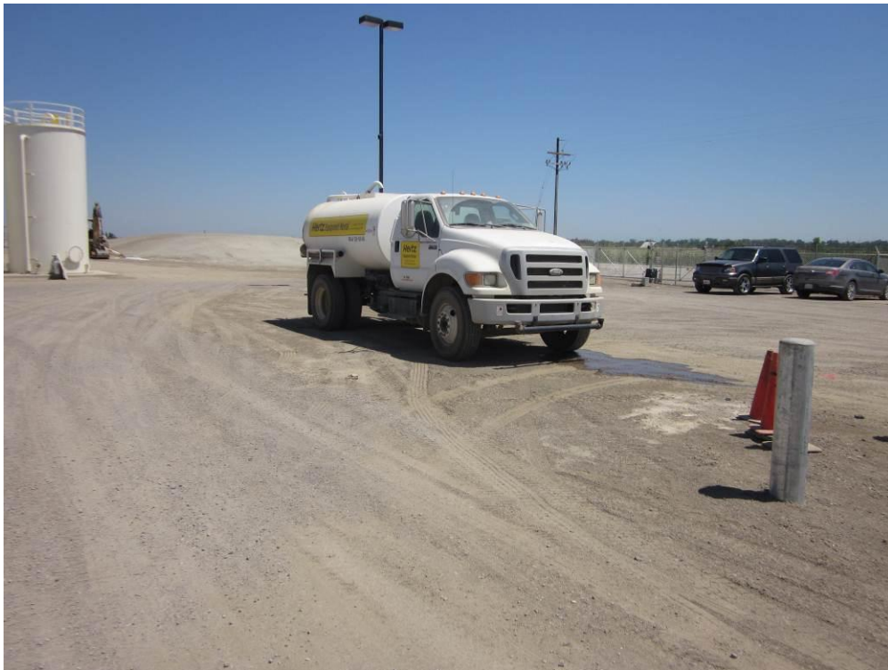
Photo 4: On-site dust at the Compressor Station site was being controlled via the use of water trucks.
