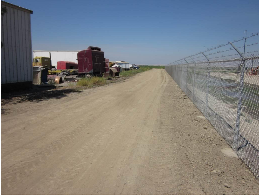
Photo 3: The silt fence along the southern boundary of the Compressor Station has been removed and the final perimeter fence installed.
